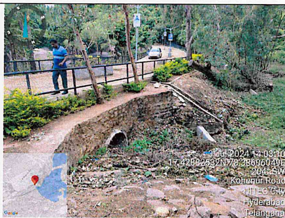
Durgam Cheruvu storm water drain inlets
