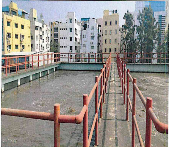
Durgam Cheruvu STP aeration tanks
