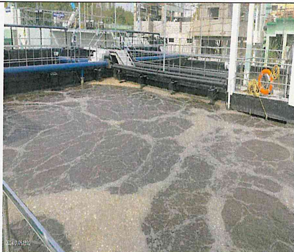
Durgam Cheruvu STP aeration tanks
